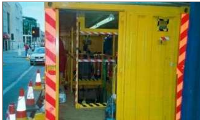
Figure 9 - HV cable jointing container
